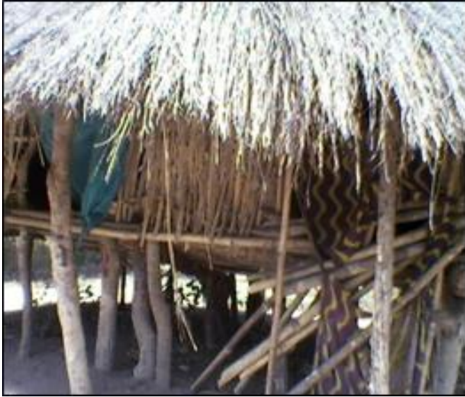
Caption: Magrete's former house, in a state of major disrepair.
